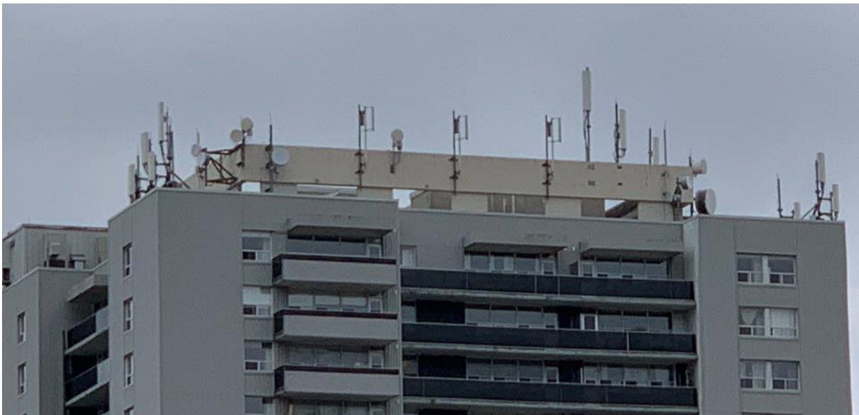
Fig 11. Sample cellular repeater station atop of a residential building
